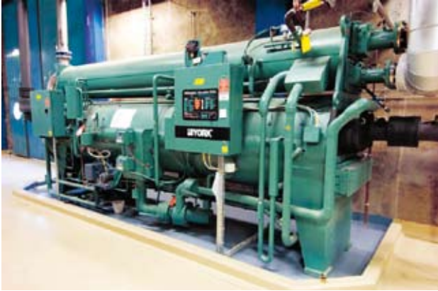
VEAB is demonstrating absorption cooling.
